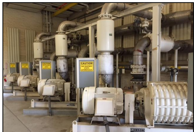
Multi-stage centrifugal blowers produce process air at the SEWRF.
