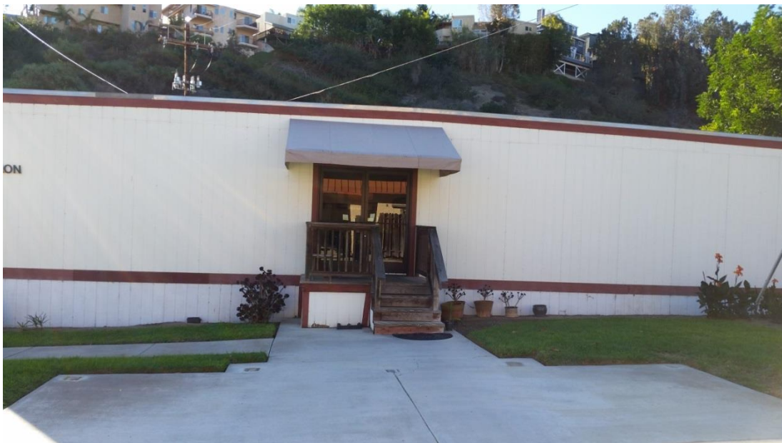
Photo 3 Non-ADA compliant Administration Building entry
