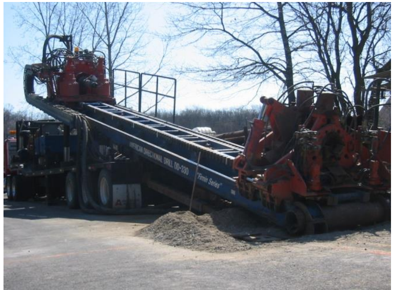
The Thornapple River Crossing project successfully installed a 20-inch water main under the river while protecting the environment and meeting all regulatory requirements.
