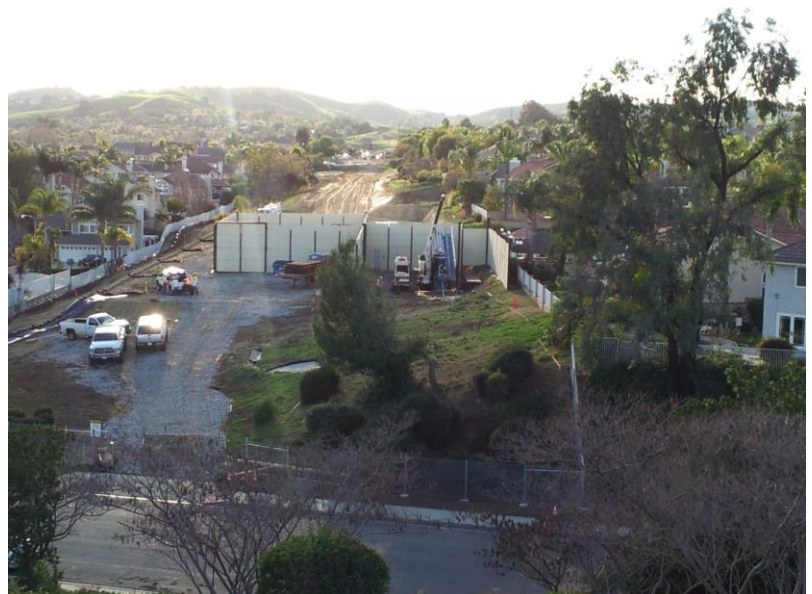
Sound walls were installed to provide mitigation to local residents during construction of the HDD for the Chino Hills project
