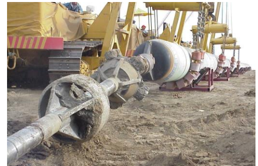
Pipe Handling Equipment
